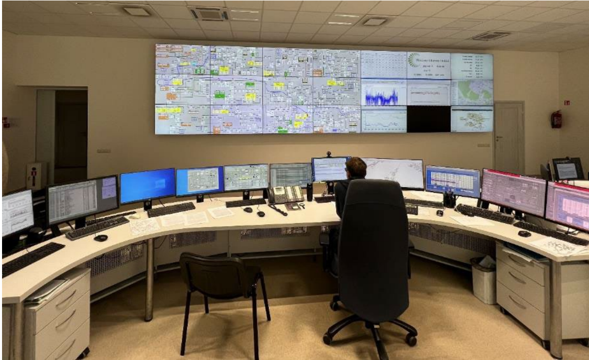
Figure 4.2. Modern network control panel installed in the Vilnius DH network dispatch centre (photo by LDHA)
