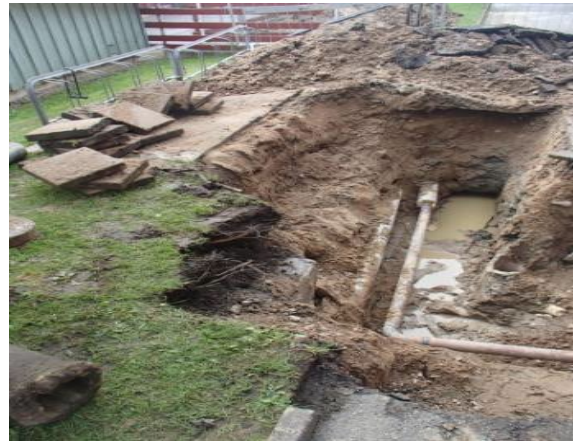
Fig 2.15. PVC type pipeline (photo by Öresundskraft AB)
