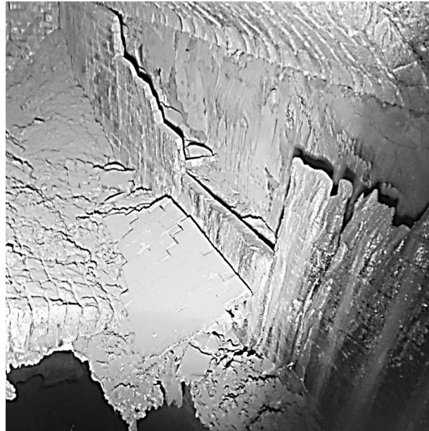
Figure 2.1. Furnace damaged by alkali bursting
