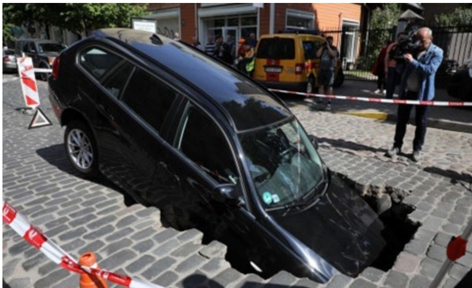
Figure 4.6. Example of soil collapse due to large rupture during pressure test (data from Quest Integrity)
