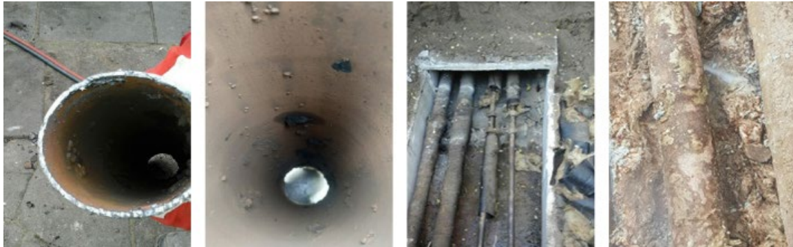
Figure 4.3. Example of internal tube corrosion and leakages (photo by AB Vilniaus šilumos tinklai)
